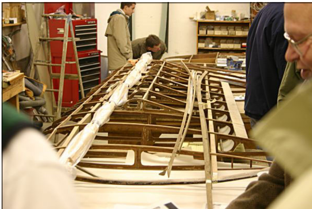
An individual wing rib — one of many — essentially intact, but in need of clean-up and regluing.
